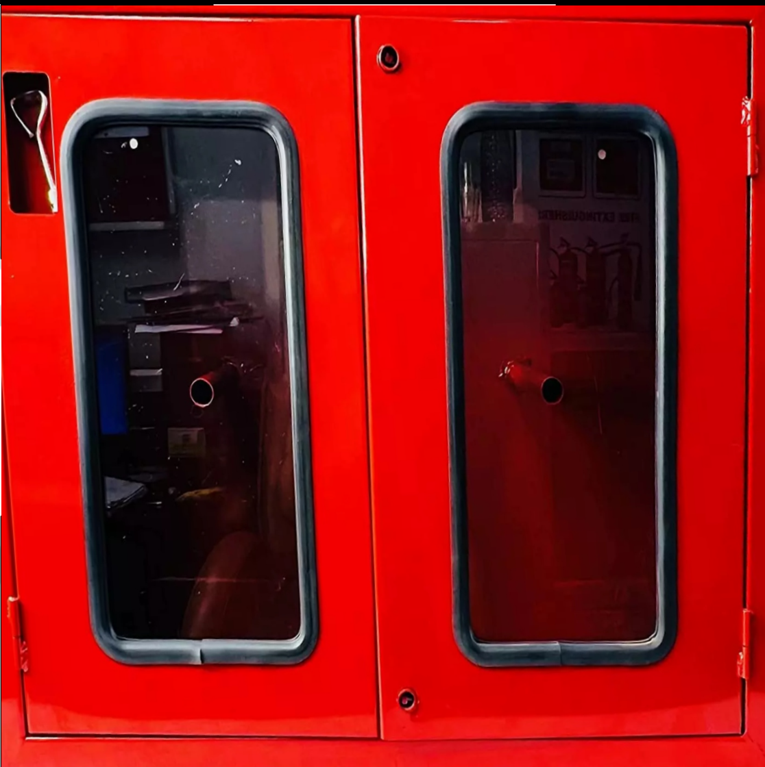
HOSE BOX & CABINET
